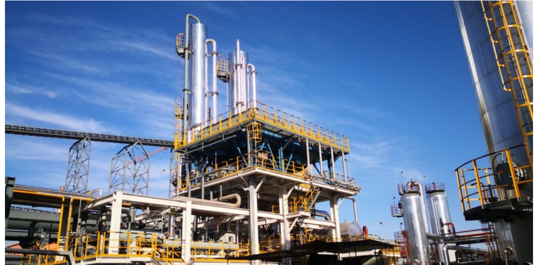
Figure 1. The world's first commercial-scale CO 2 -to-methanol plant has started production in Anyang, Henan Province, China. [01]
